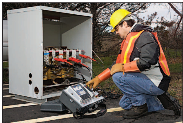
TTR330 shown testing a pad mount three-phase transformer
